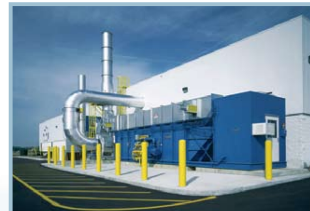
RTO: Regenerative Thermal Oxidizer
