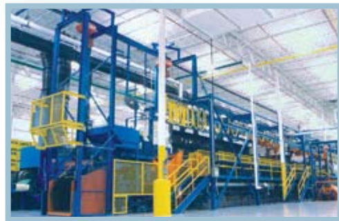
Phosphate Pre-Treatment Line
